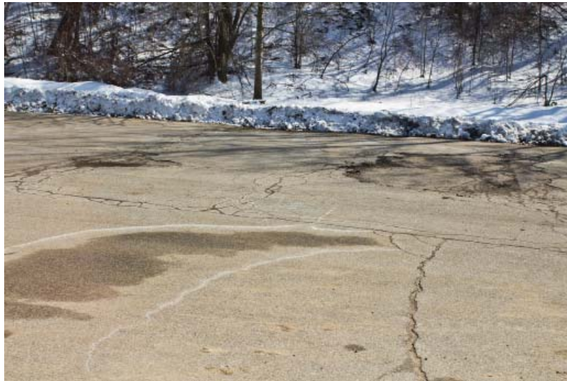
Safety issues exist, such as this deteriorated blacktop on the Gossler Park playground
